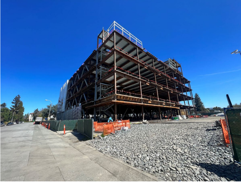
CoreSite's SV9 240,000-square-foot data center, located at 2915 Stender Way, is under construction at the Santa Clara campus. The structural steel and concrete pours are now complete.
