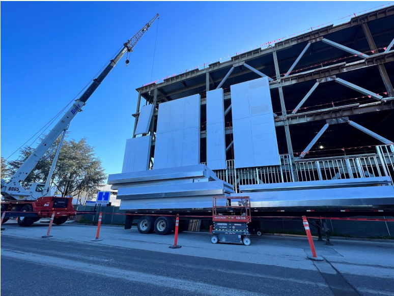
CoreSite has begun the installation of the exterior skin systems with building dry-in planned by Summer 2023 for its SV9 facility in Santa Clara, California.
